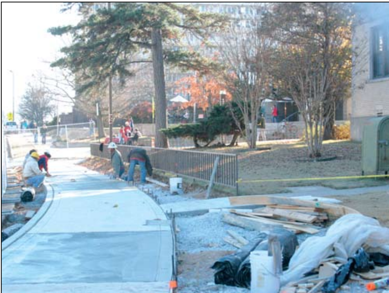
Construction workers replace part of the sidewalk near Gibson Hall. Various other construction projects are planned to be completed in 2009 and 2010.
